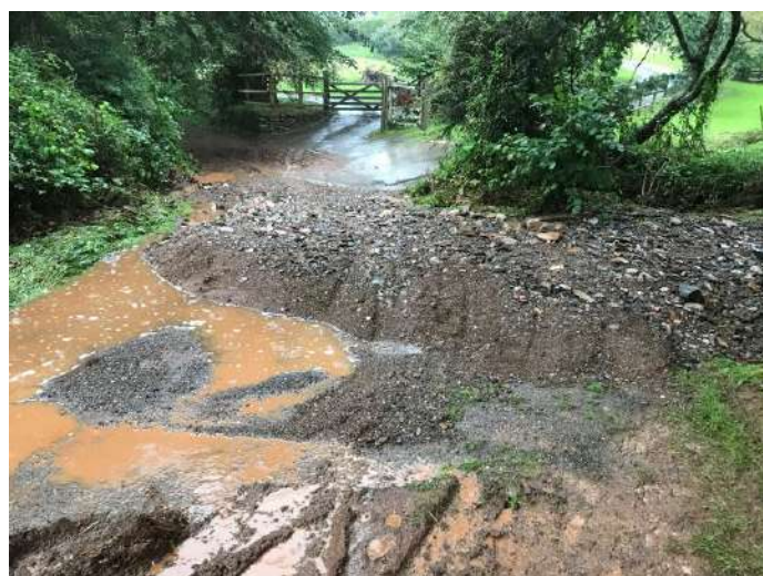
Wash down from watery lane which blocked the Belsford hamlet's only road
