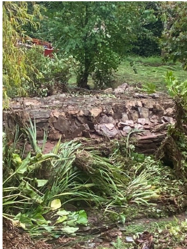
Collapsed wall at Ashbrook Cottage
