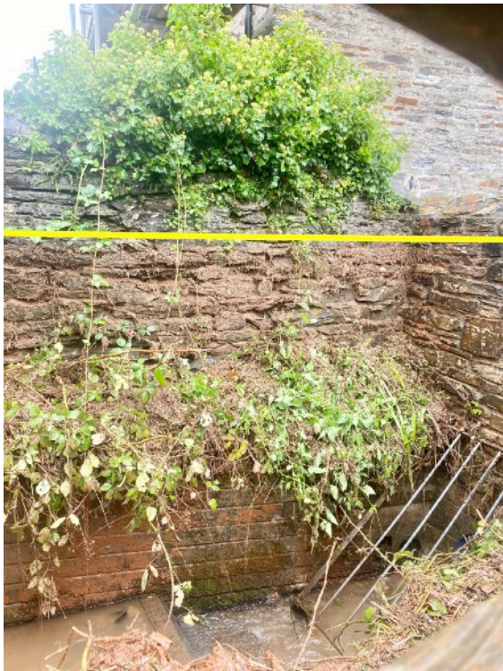
Inclined grating over the culvert
