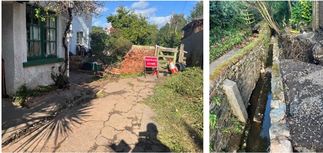
Figure 6.3. Damage caused to the footpath in Kenton.
