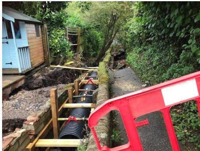
Figure 6.4. Temporary works on the watercourse to support the footpath in Kenton and maintain flow in the brook.
